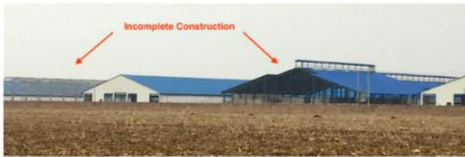
Incomplete construction at Huishan Wufeng Dairy Erdao Hezi. Photo by MWC investigator.
